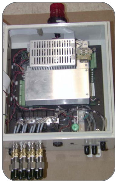
Interior, Chemgard Gas Monitor
